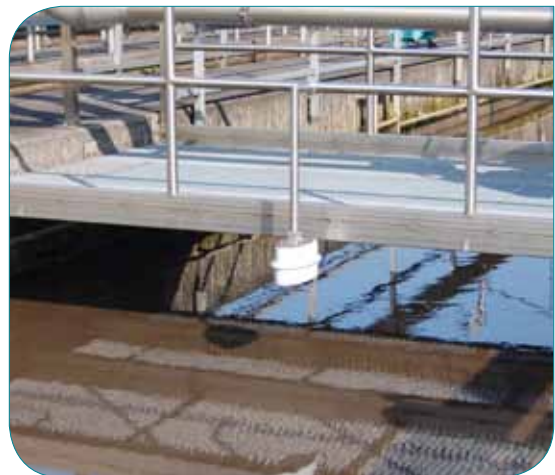
Pic: SQ-Sensor installed
